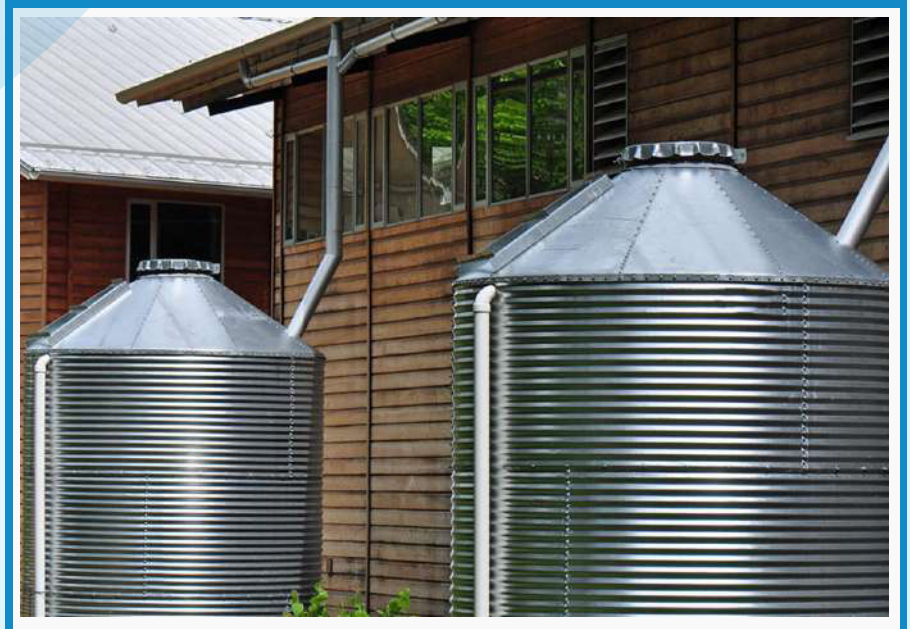
Rainwater Harvesting System
